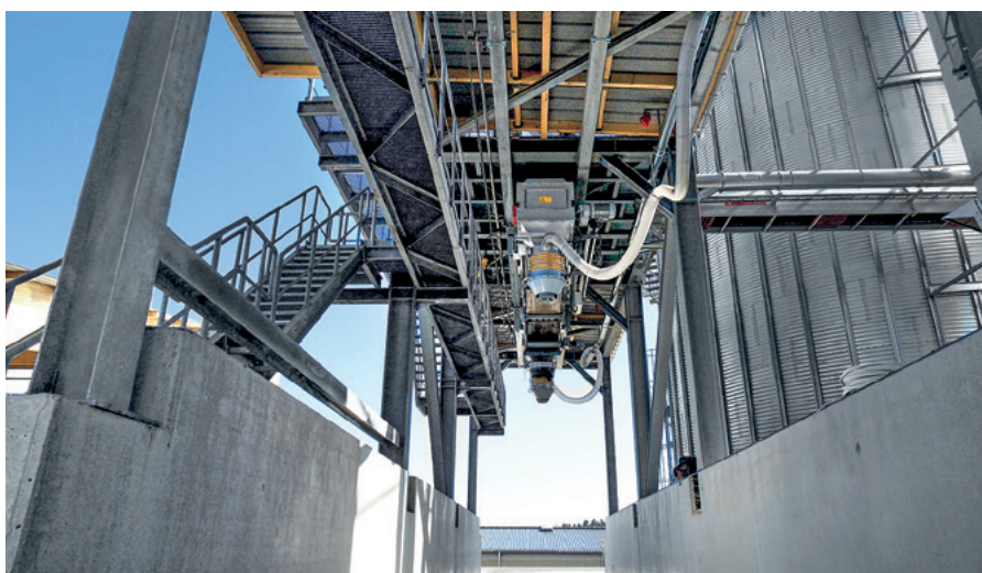
Truck loading station with mobile conveyor belt
